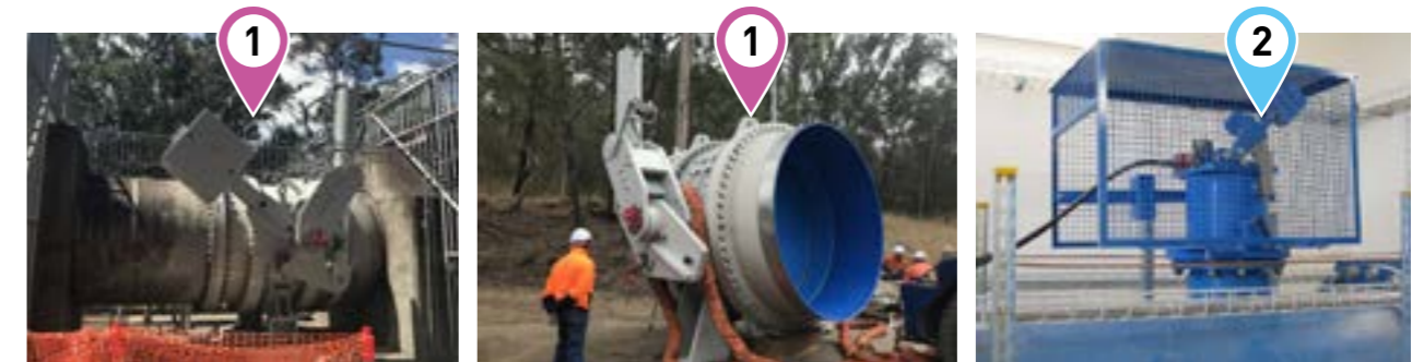
REAL-LIFE TALIS EXAMPLES OF SAFETY VALVES IN TRANSMISSION PIPELINES.
